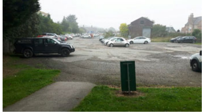
The Station Car Park. Significant up-grade work, including lighting, is needed.
