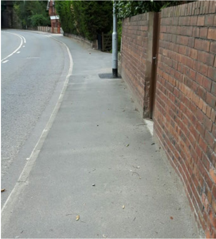
Above: The narrow footway on the north side of Main St looking towards the railway bridge and FP33.
